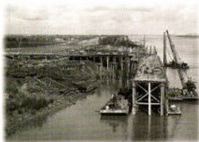
General Cargo Dock No. 1 under construction. It was the first facility to be completed at the port.
